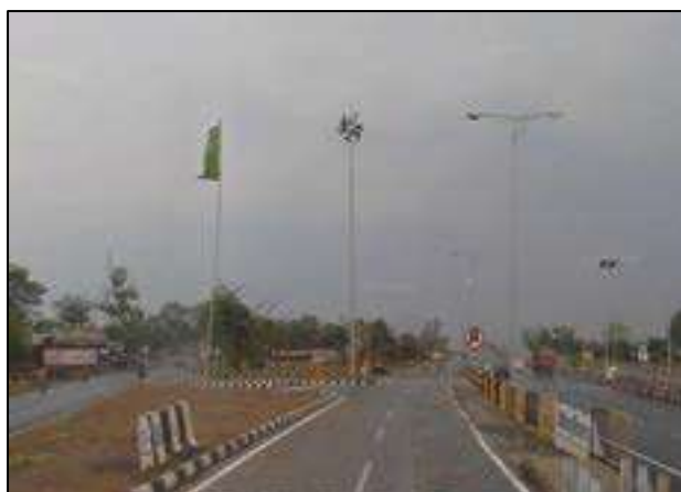
High Mast Light at 353+950
